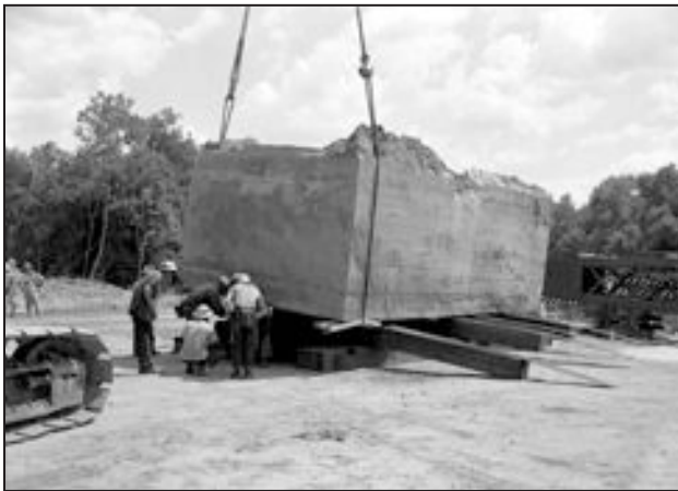
100-Ton Concrete Block Used for River Dock Construction, June 25, 1952, SRS Negative M-1054-07
