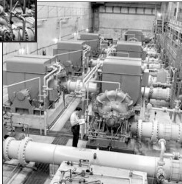
Interior View of 681-1G Pump House, March 20, 1956, SRS Negative DPSPF-3178-3-11
