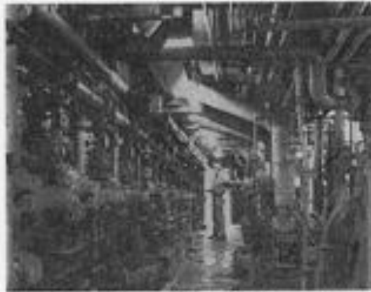
Desalination units and control valves, checked here by Thomas Ables, H Area, purify the water before it is added to steam boilers.
