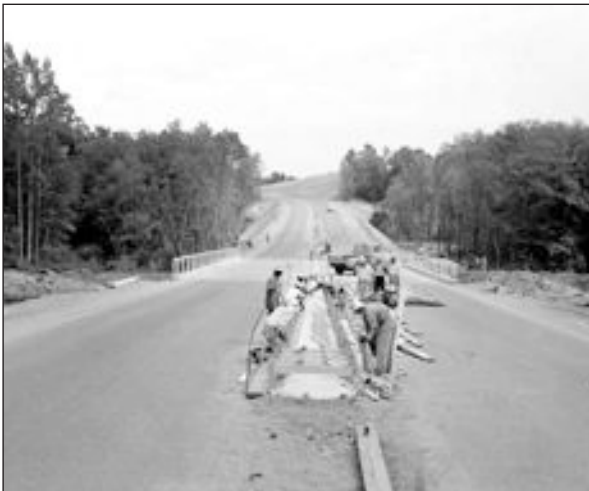
Preparation of Cement Forms for Three Run Road, September 12, 1957, SRS Negative M-285-06
