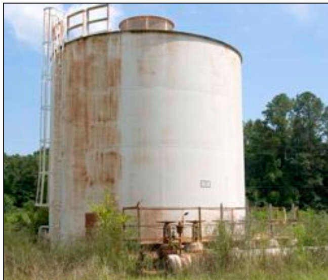
Cooling Water Surge Tank, July 2009, SRS Negative 0901178087
