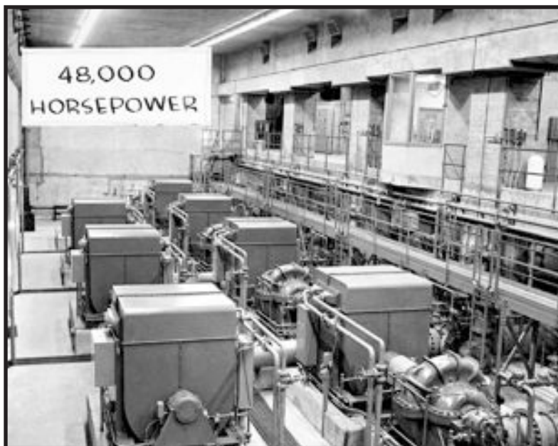
Interior of 681-1G Pump House, date unknown, SRS Negative M-3193-01
