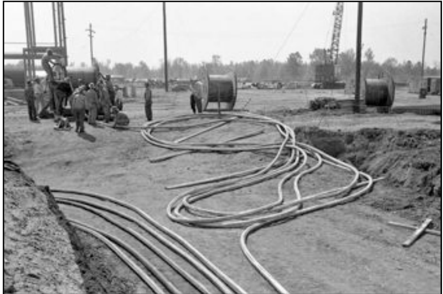
Lengths of Electrical (Possibly Supervisory Control) Cable in D-Area, April 9, 1952, SRS Negative DPESF-732-05
