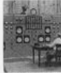
Joe Hinesman looks check on control board in one of the main pumphouses between reservoirs and production areas.
