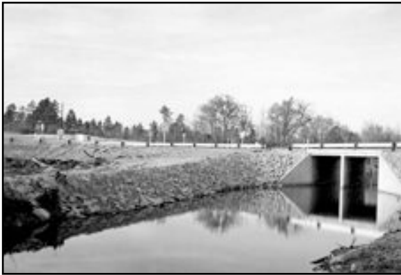
Road, Culvert and Rip-rap at 39 and G Roads, December 17, 1952, SRS Negative M-1733-01
