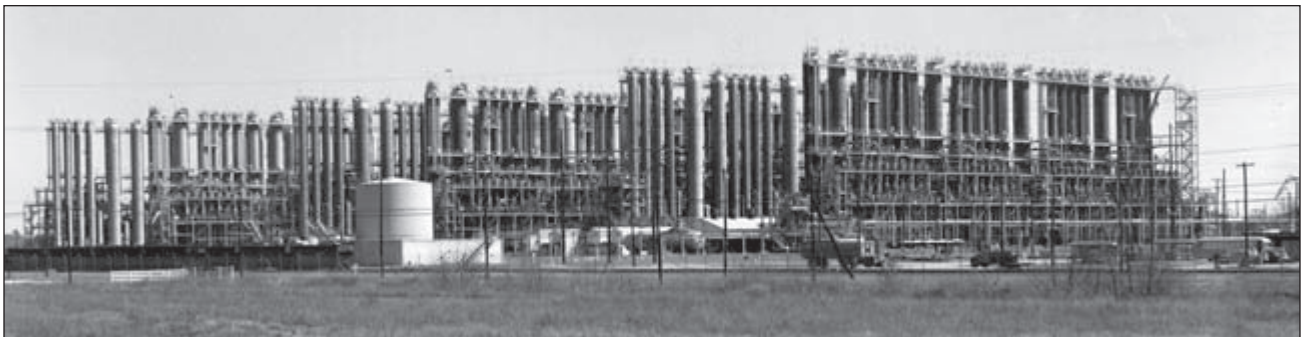
Building 402-D, Tank Farm. Views showing railroad-side facility (above) and "car spots" (opposite) after completion. Courtesy of SRS Archives, negatives 3142-2 and 402.
