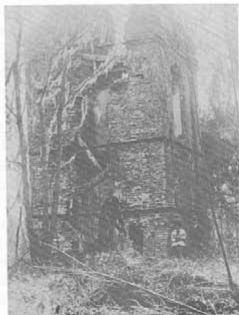
Three sets of steel straps, put in place through the efforts of the National Society of Colonial Dames, held the ruined tower together for about fifty years.
