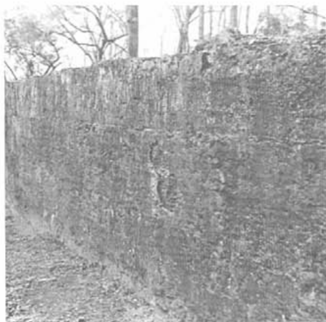
A close look at the fort shows the layers of tabby and the oyster shells that make up the material. Carolinians commonly excavated old Indian shell mounds for the thousands of bushels of shells required in tabby construction.
