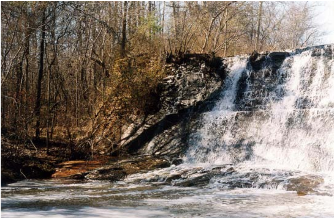
Figure 21. Photograph of West End of Dam. Peters Creek will be rerouted to the left of the dam through the old spillway.
