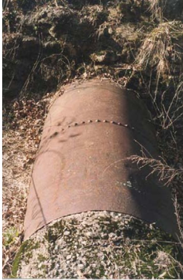
Figure 27. Photograph of Riveted Iron Pipe Through Dam Showing Transition to Concrete Flume.
