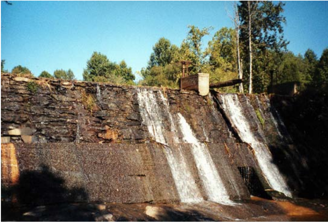
Figure 20. Photograph of Dam Showing Poured Concrete Base and Floodgates. View to the north.
