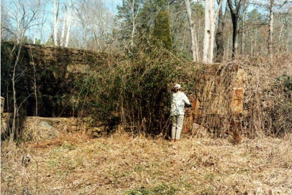
Figure 23. Southwest Side of Mill Building Showing Opening, Possibly for Driveshaft to Turbine.
