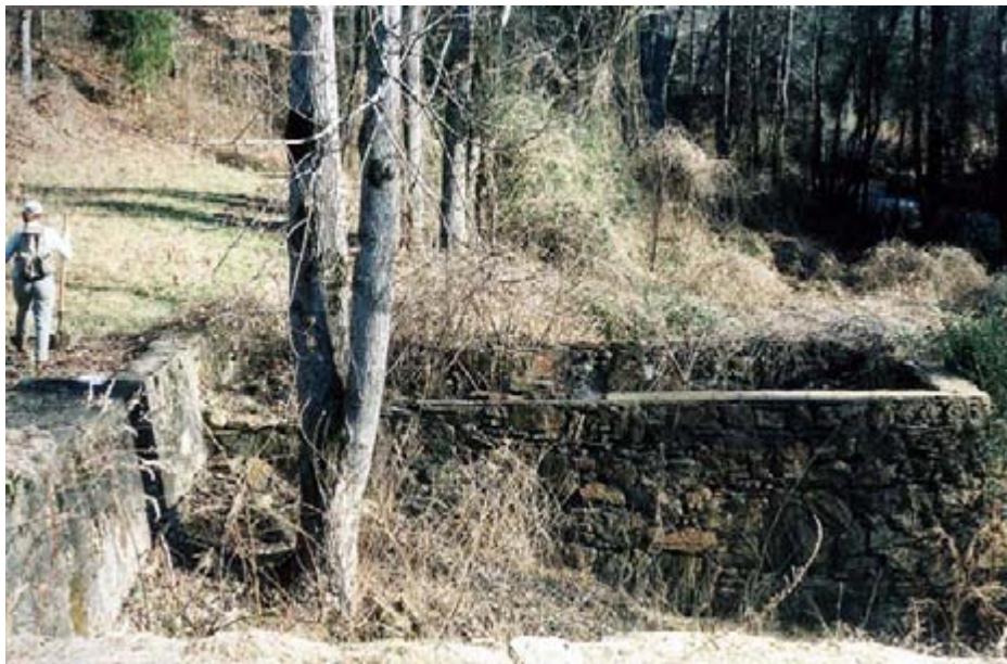
Figure 22. Foundation of Mill Building with Bulkhead/Retaining Wall to the Left. View to the southeast.
