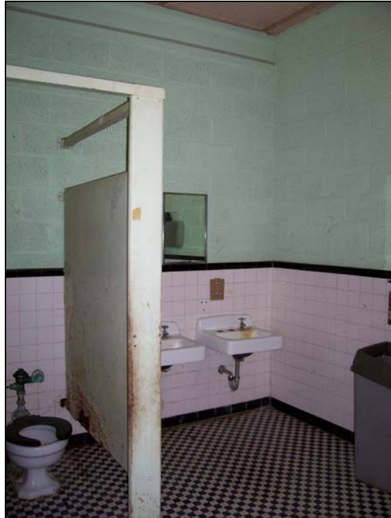
Figure 13. Sinks in girl's bathroom at Bucksport Elementary School.
