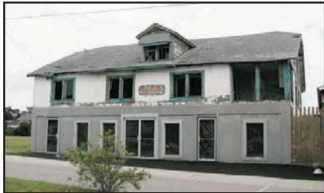
32B. Loss of Significant African-American Sites Through Decay or Incompatible Renovation Techniques (Site 2494)
