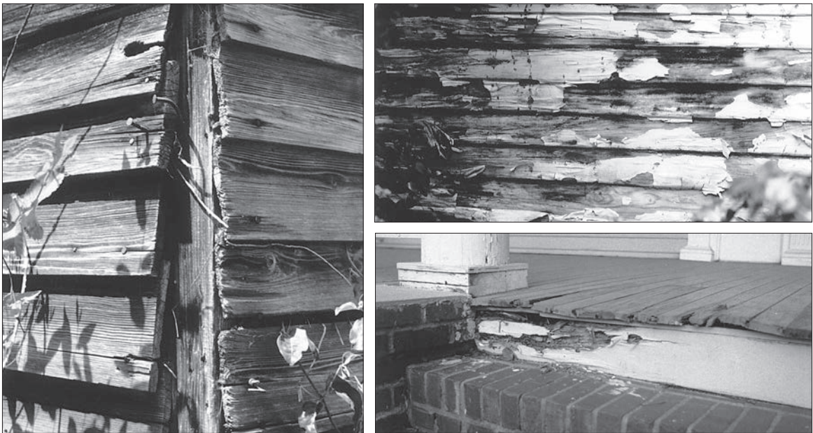
CLOCKWISE LEFT TO RIGHT: Wood siding requires painting to protect it from both the weather and the sun. This heavily weathered siding, which is missing its cornerboards, shows the results of long exposure to the sun — ultraviolet light destroys the wood. / This is an example of a serious moisture problem in a wood-sided building. The peeling paint and dark mildew stains are a sure indicator of moisture in the siding, and there are signs of dry rot as well. The source of moisture could be improperly-installed insulation, a leaking gutter or downspout, or leaking plumbing inside the house. / Wood porches are exposed to the weather and tend to be susceptible to deterioration. In this case, dry rot has caused a face piece, and probably structural members behind it, to lose its physical strength and crumble away. Note also the buckled floorboards, a sign that they are absorbing excessive moisture. Wood with dry rot must be replaced as soon as it is noticed so the rot will not spread.
