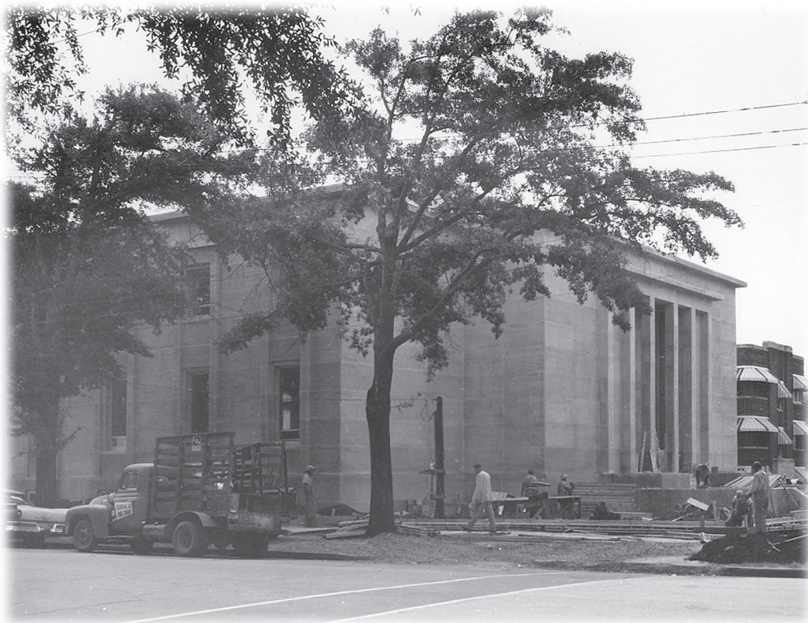
The Archives building at the corner of Senate and Bull streets under construction in 1959.
